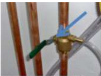
Water valve in "off" position
