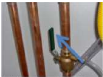
Water valve in "on" position
