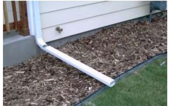
This is the downspout extension. Keep it in this position so roof rain water drains away from the house.
