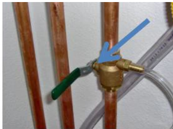
Water valve in "off" position
